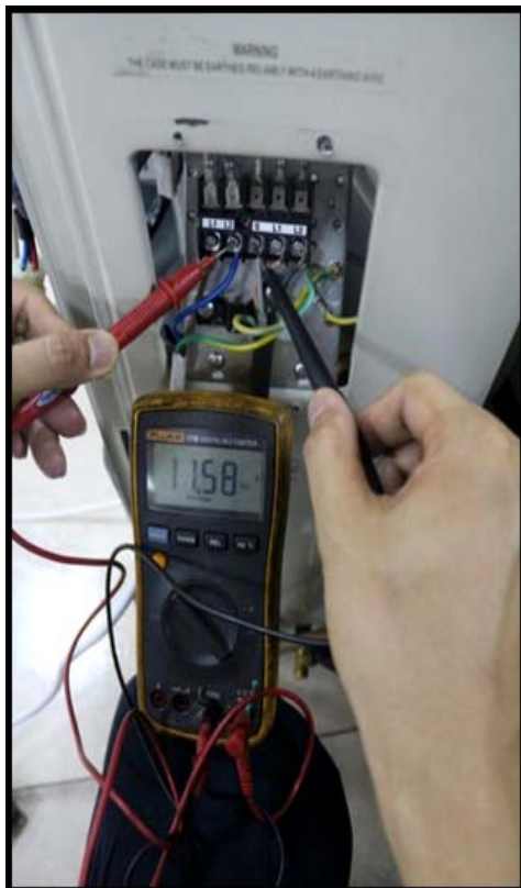
Fig. 32 — Test the DC Voltage
